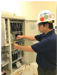
Shop Testing of Tekran 3300Xi HgCEMS
