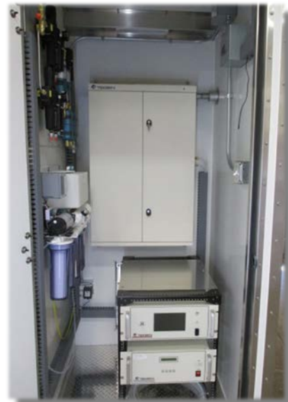
Cabinet Interior showing the Tekran 3300Xi "Next Generation" HgCEM System
